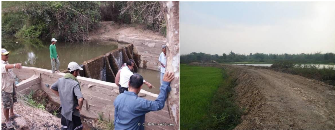
Figure 8. Dam and weir construction at target villages to improve water management and availability
